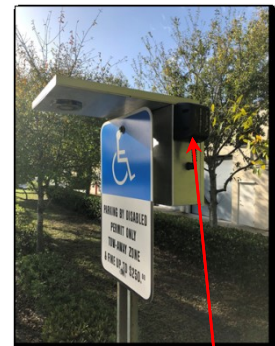
Figure 2 Retrofit Volt Meter Solar LED Bus-Stop
